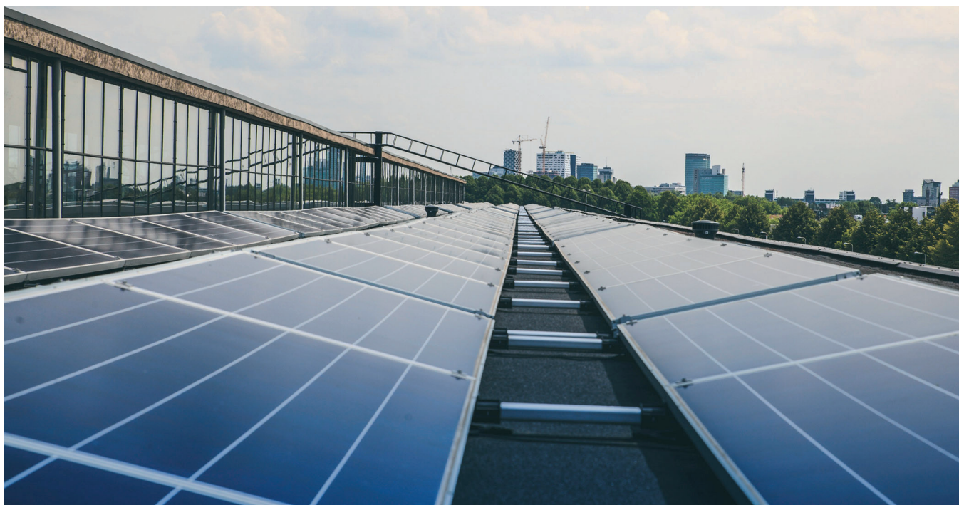
Rooftop solar panels
